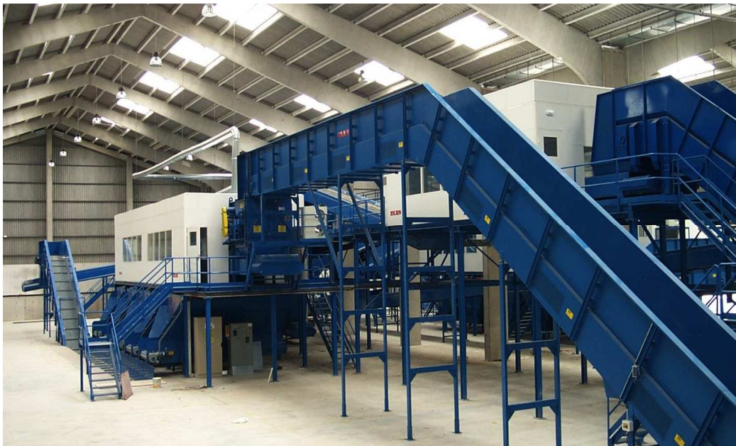
Waste Recycling plant
